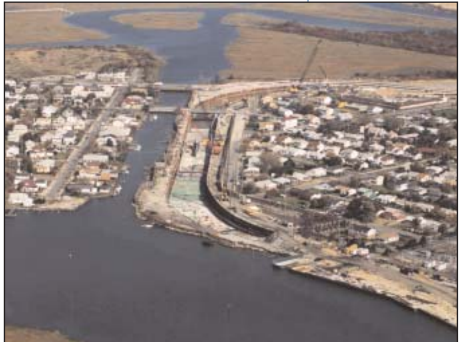
The Atlantic City Brigantine Connector cut and cover tunnel section was excavated parallel to the Penrose Canal to a depth 30 feet below sea level.
