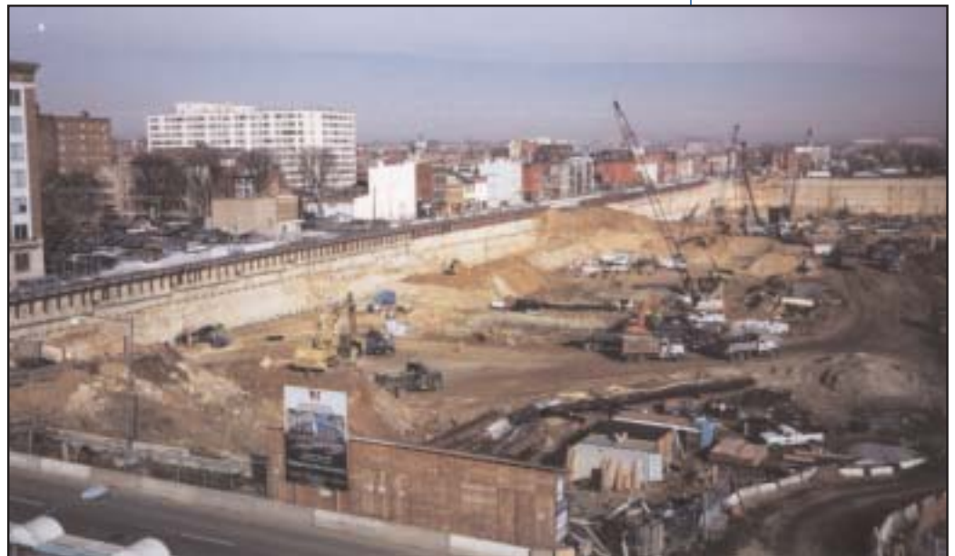
Massive excavation within the slurry wall confines cover an area previously occupied by six city blocks.
