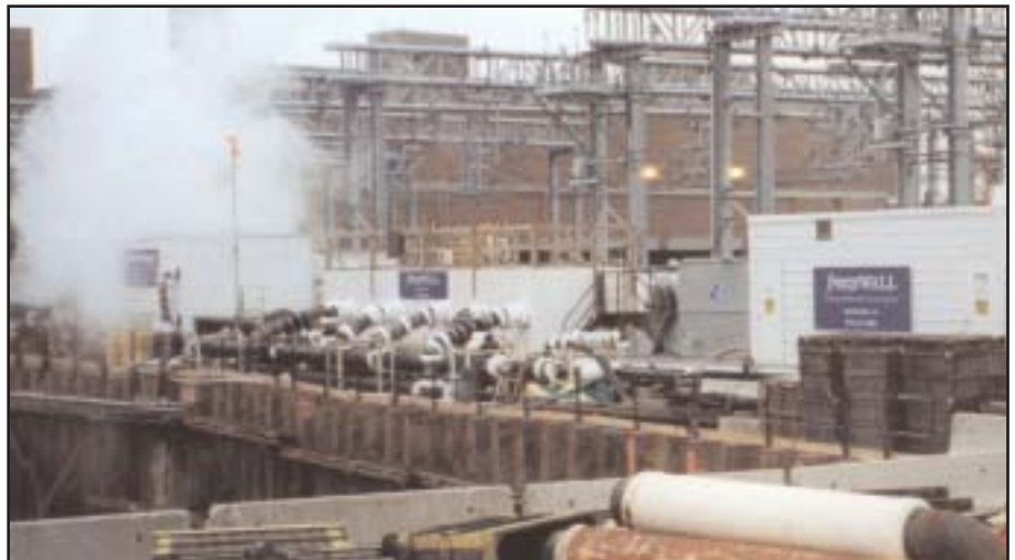
Chilled calcium chloride brine was circulated through more than 2,000 freeze pipes.
