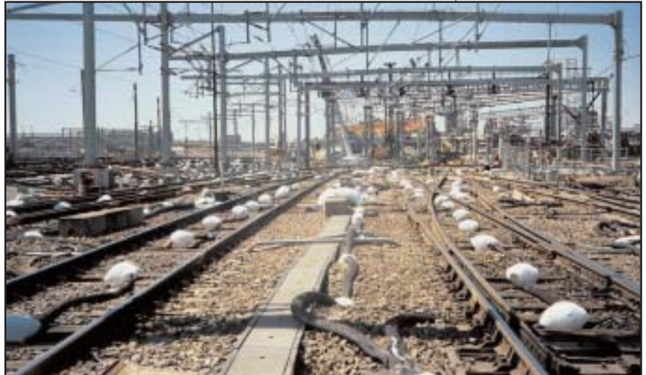
The operating ground freezing system stabilized the ground and rail lines during construction of three tunnels comprising the Interstate 90 Extension.
