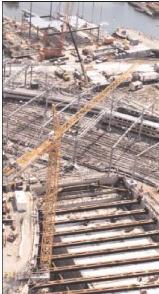
Three massive concrete boxes were jacked under these portions of the rail lines.
